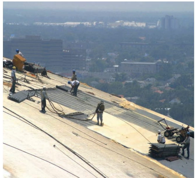
Photo 5: Spray foam application. New fully adhered roof insulation and integral air barrier.
