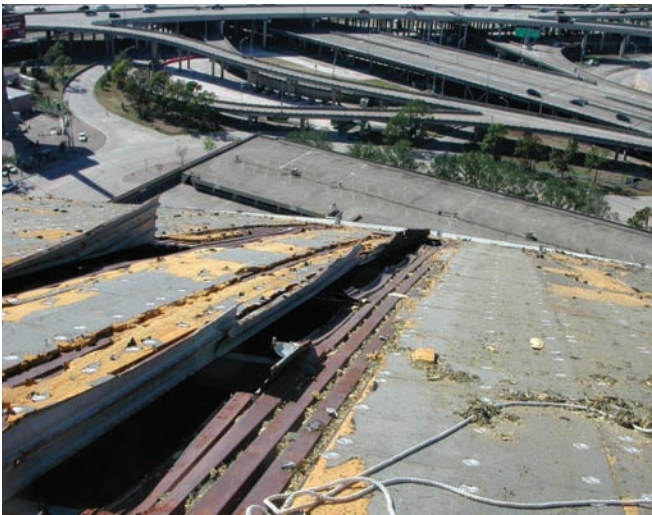
Photo 4: Superdome roof damage. Missing membrane and exposed rigid sheet insulation. Note the mechanical connectors. The membrane was adhered to the top of the sheet insulation boards and to the mechanical connectors. Also, note the metal deck and the flutes that allowed lateral airflow and lateral water migration.
