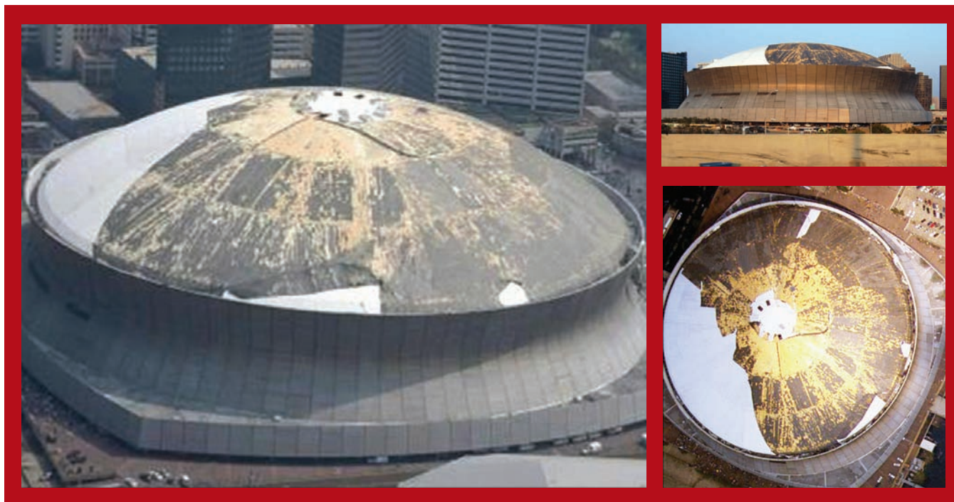
Photo 1: This never should have happened. The Superdome's roof membrane is missing after Hurricane Katrina in 2005.
