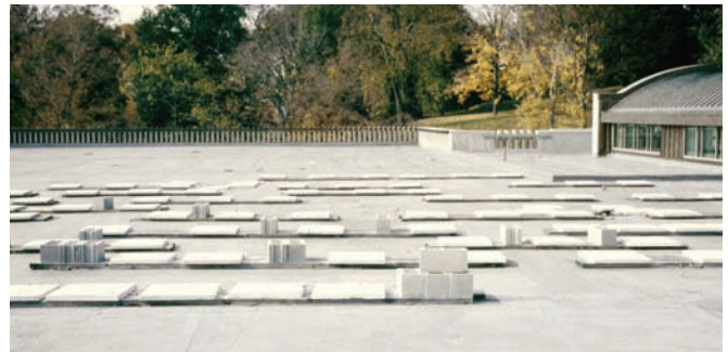
Photo 3: Fluttering membrane fix. "I'll fix that darn moving membrane. Get me some pavers and blocks."
